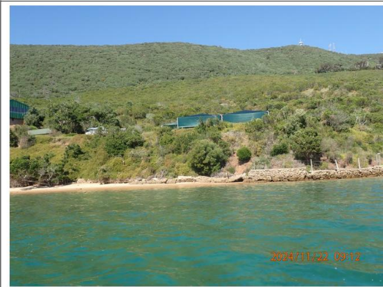
Fig. 18. Area of proposed Managers Cottages, viewed from estuary. Note damaged sea wall below and erosion on embankment. Erosion is further evident on the embankment below the exiting garages, on the estuary side.
