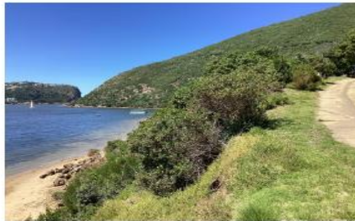
Fig. 13. Embankment close to estuary, below access road to existing garages, site visit 17 October 2023. This embankment previously suffered erosion and was rehabilitated.
