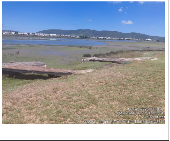
Fig. 10. Knysna Sea Cadets’ slipway and jetty in need of repair and upgrading.
