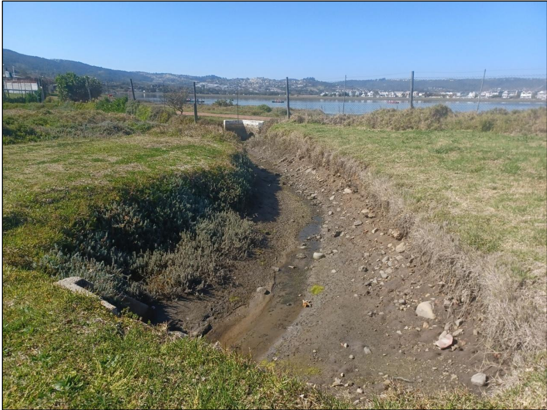
Plate 5: A photograph taken of one of the drains showing active saltmarsh habitat where the drain is below the HWM, note the right bank where the vegetation is mowed and appears to have been damaged
