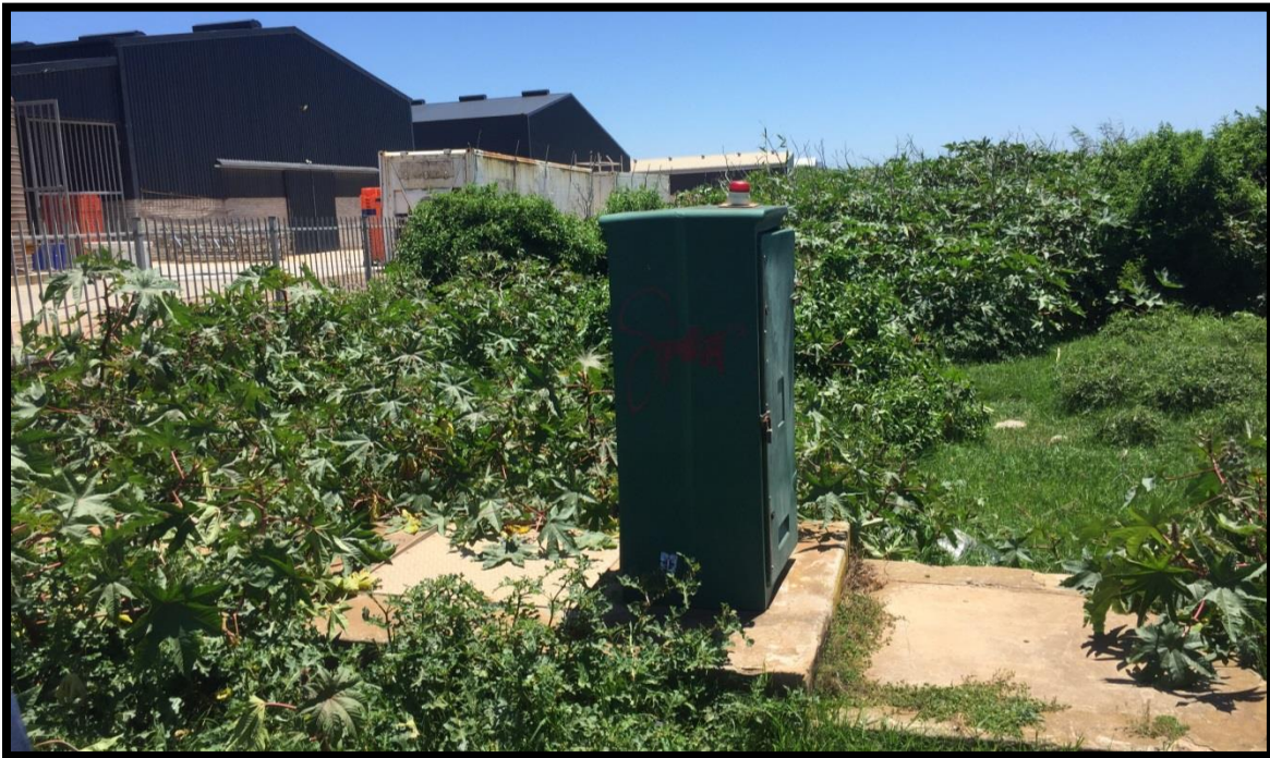
Figure 4: Tarragona Sewer Pump Station
