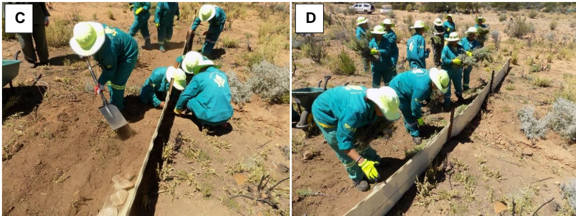
Figure 15. Installation of the soil erosion control fence. A: Installing the standards and wires and preparing the trench. B: Fitting the geotextile, tying it on with wire. C: Filling in the trench over the geotextile. D: Applying a mulch against the completed fence (Photos courtesy Ken Coetzee).
