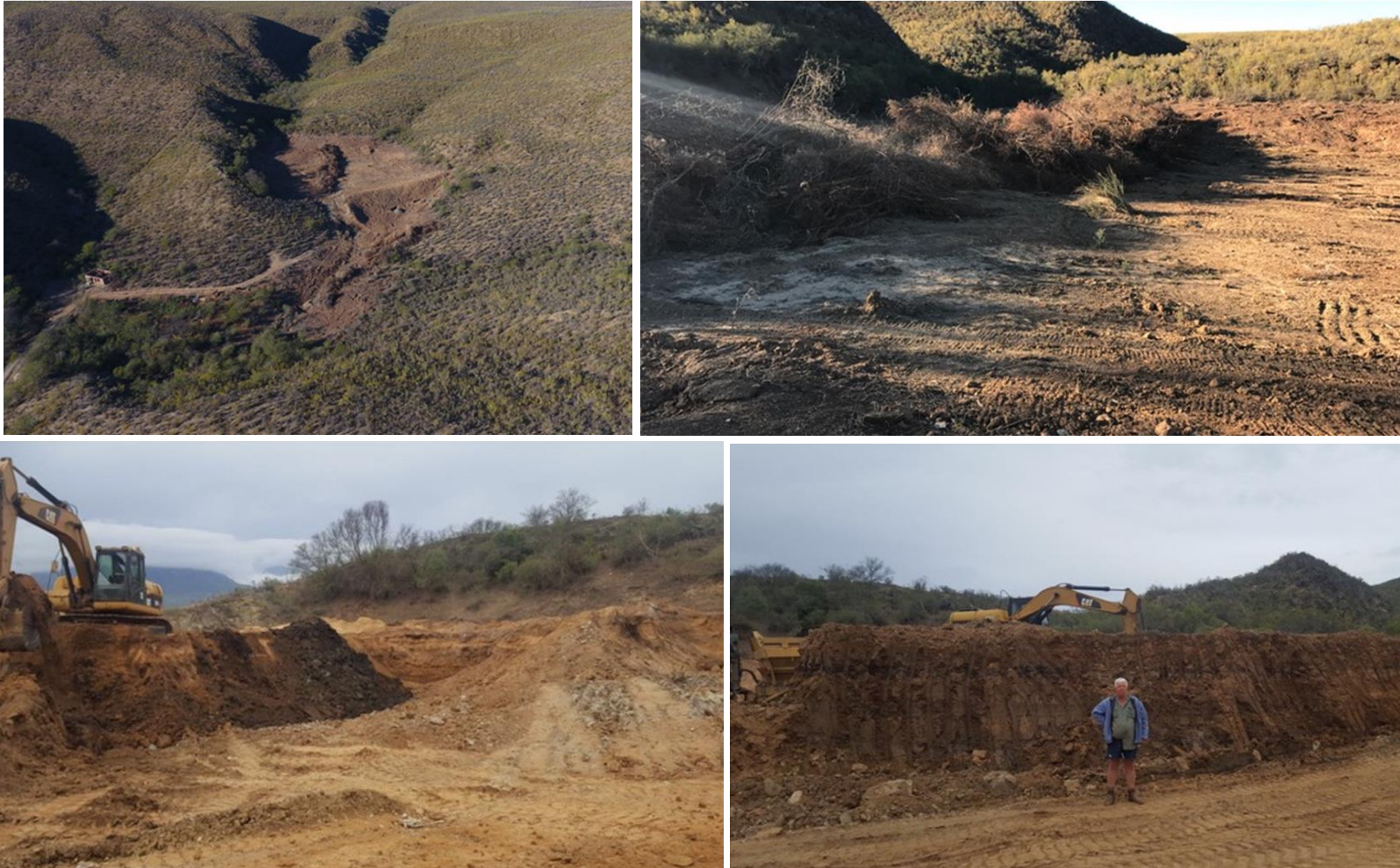
Figure 17. Photos taken during the construction phase of the dam enlargement by the landowner (J.C. Jansevanrensburg; September, 2017).
