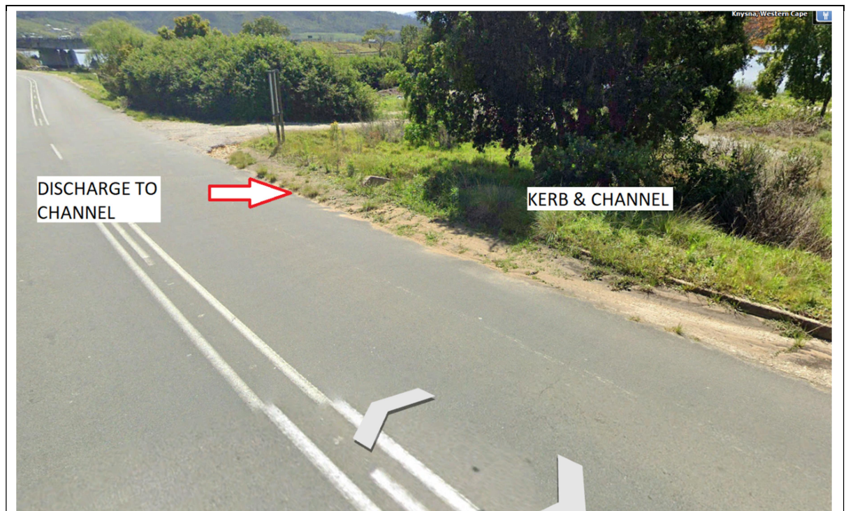
FIGURE 6: EXISTING KERB AND CHANNEL IN DIV. ROAD SILTED UP
