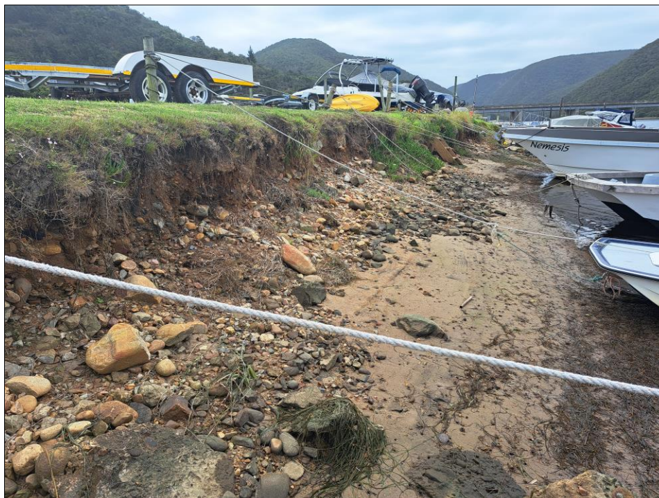
Figure 1: Photograph showing erosion of the bank.
