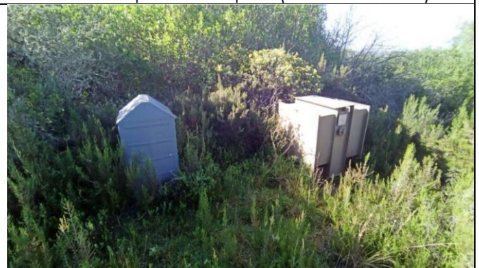
17. Electrical boxes / "housing" on the eastern boundary of Erf 1058 (Dr. Peter Nilssen).
