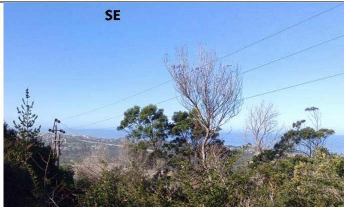
21. The overhead power line crossing Erf 1058 (Dr. Peter Nilssen).
