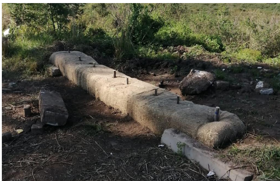
Figure 8. Example of hay bales bound together with hessian / jute and staked to prevent surface runoff into the adjacent wetland.
