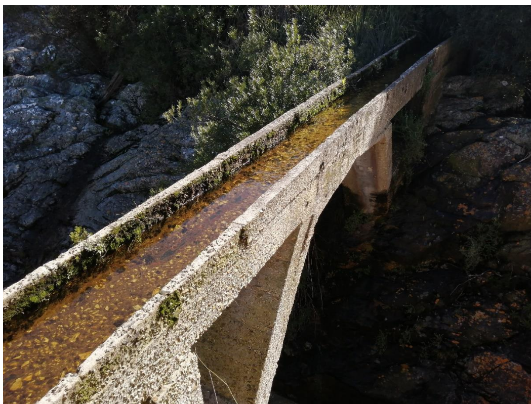
Figure 3: Photograph of the aqueduct that diverts water out of the Rondebosch River and into the furrow system.
