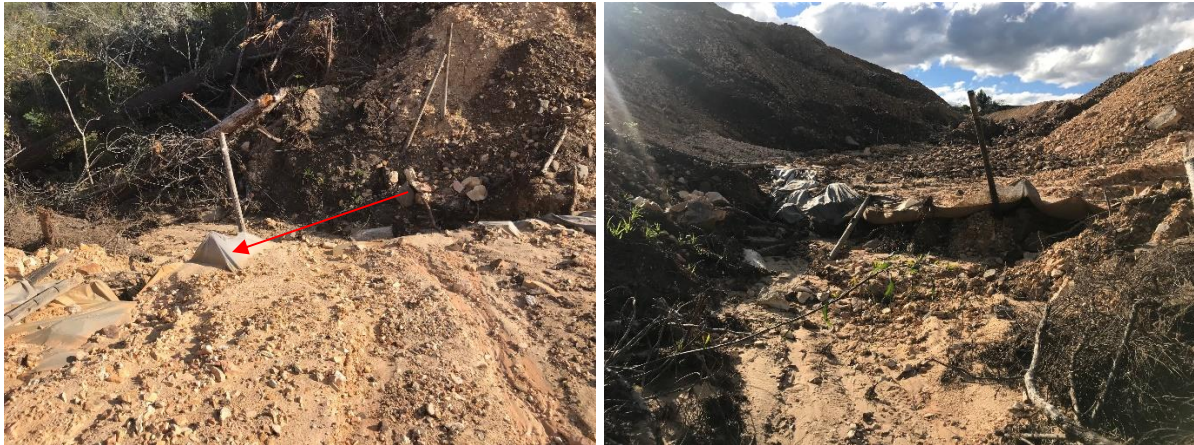
Figure 2. Photo showing the overwhelmed silt fence (indicated by red arrow) from the upstream (left) and downstream (right) perspective.
