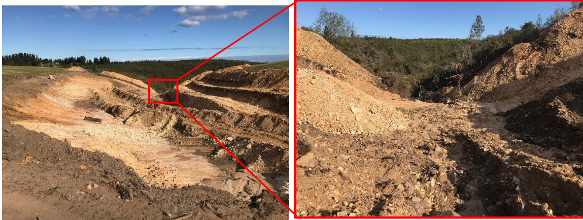
Figure 1. Photos of the excavated dam area and enlargement of the 'outflow' leading to the watercourse below.
