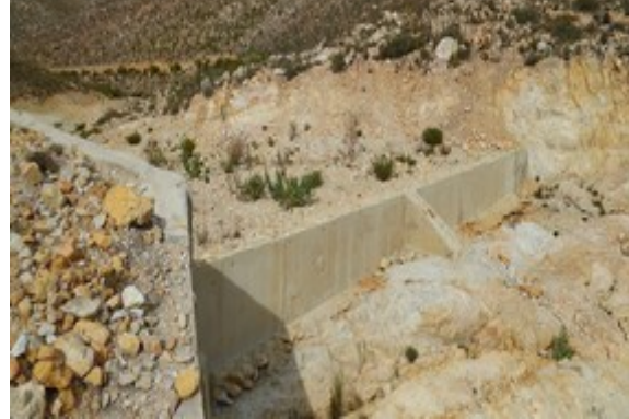
Figure 9: Typical bywash spillway with concrete end sill and retaining wall against fill embankment
