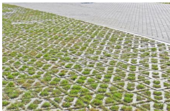
Figure 12. Example of grass pavers combined with conventional paving in a parking lot.
