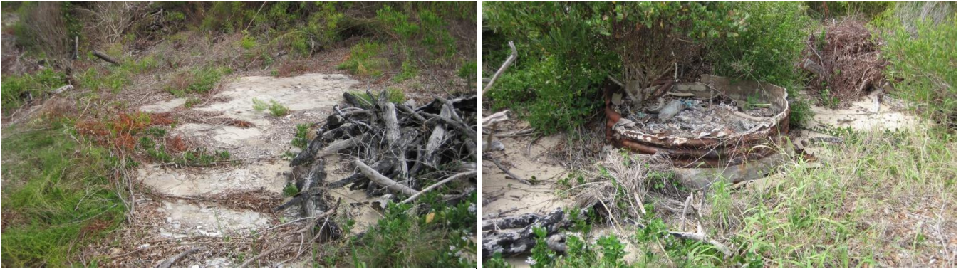
Plate 20: Concrete slab at D002. Plate 21: The remains of a small water tank at the one end of the slab.
